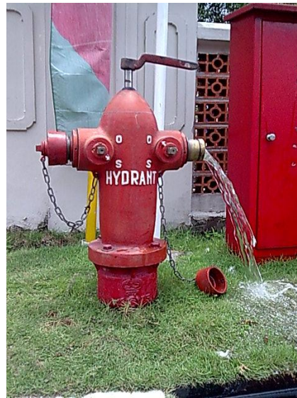
Gambar Hydrant terpasang
